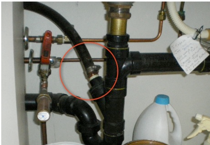
Drain line connecting under kitchen sink
